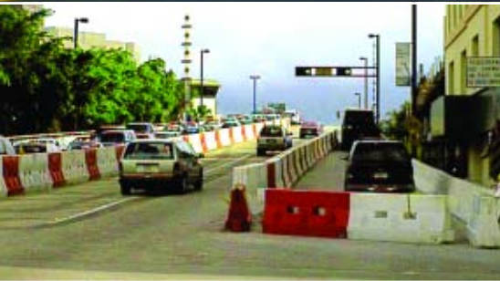
Longitudinal Channeling Barricade
